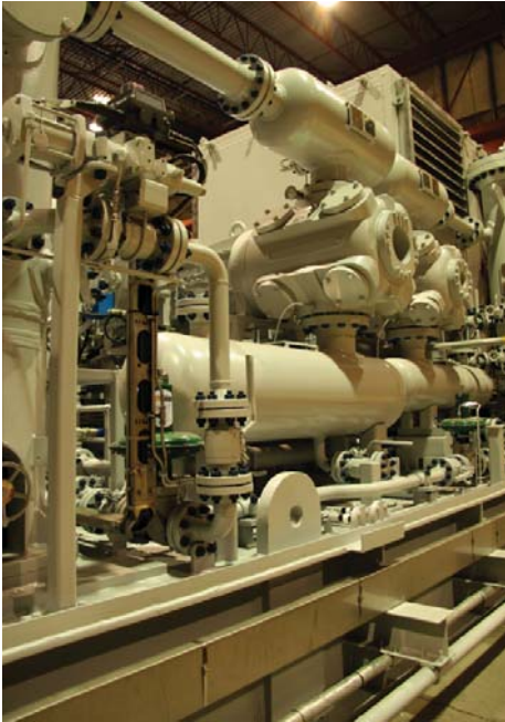
Compressors are used to feed a constant flow of compressed gas, usually air to the entire network of pneumatic tools and operations within the factory
